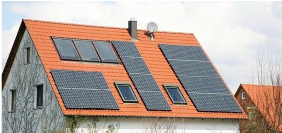
Photo 2: Solar panels on the roof of a residential building.
