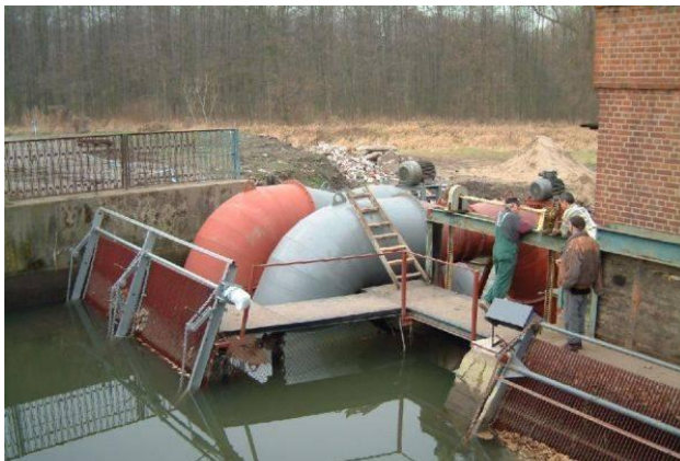
Photo 4: Small hydroelectric power plant.
