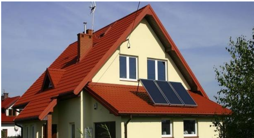
Photo 1: Flat-plate collectors on the roof of a residential building.
