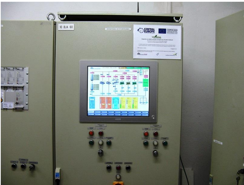
switchboard - the interface to the virtual power plant
