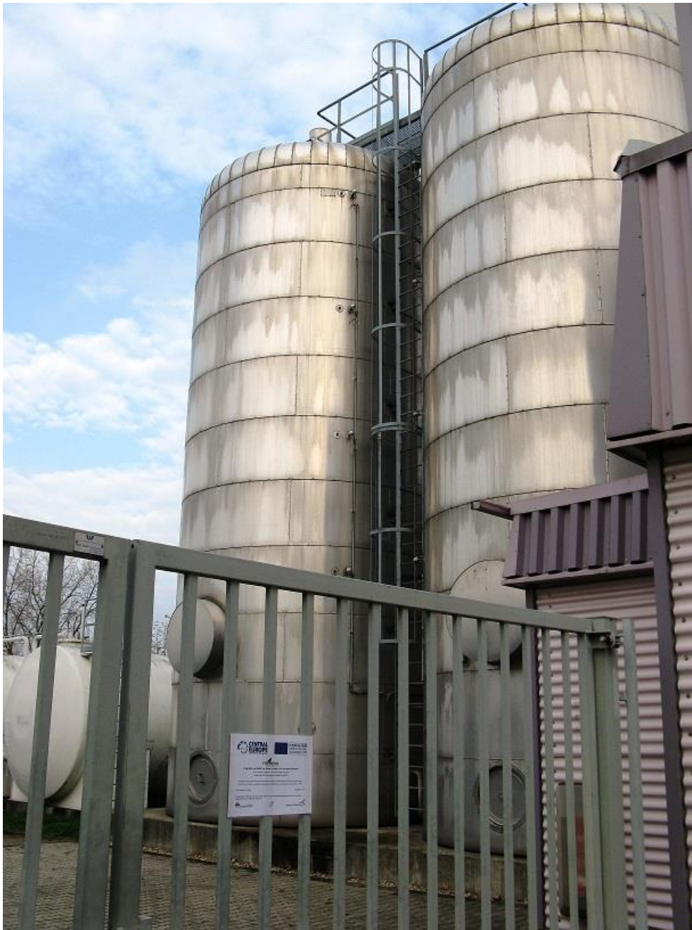
thermal storages for the teleheating system
